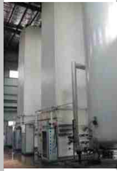
AIR SEPARATION UNIT
