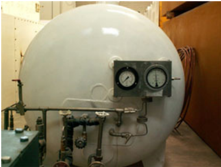
LIQUID OXYGEN CRYOGENIC STORAGE TANK
