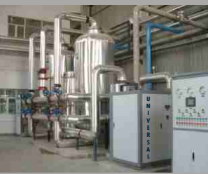
Air Purification System
