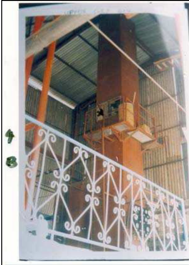
Leakage in Cold Box made from copper
