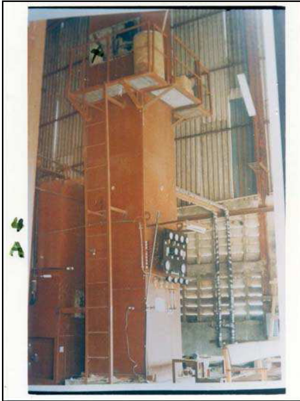
Leakage in cold box due to explosion of Copper line.
